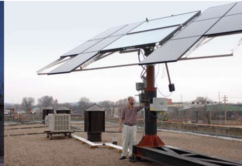
Solar panels on the roof of the University of Louisville's Sackett Hall
