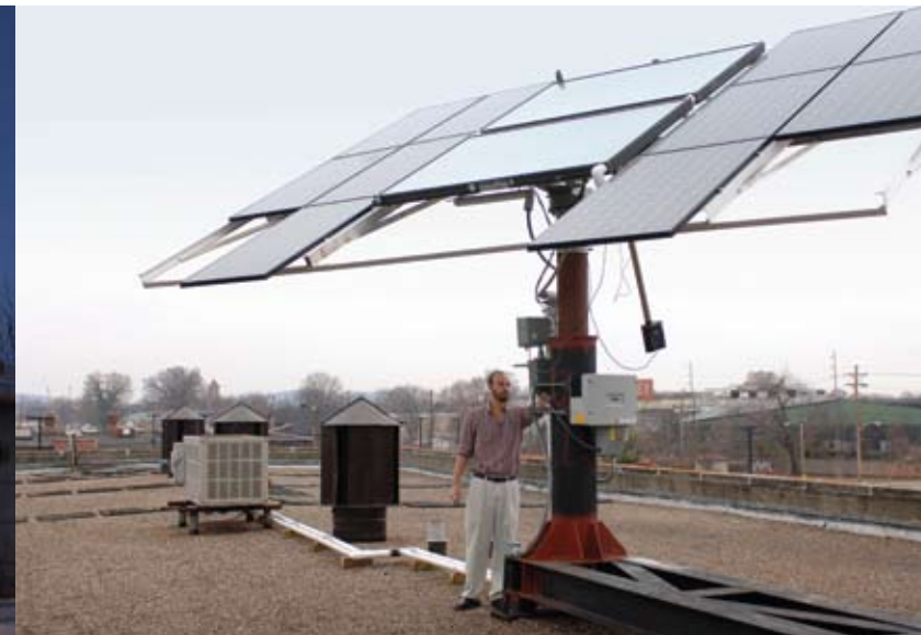
Solar panels on the roof of the University of Louisville's Sackett Hall
